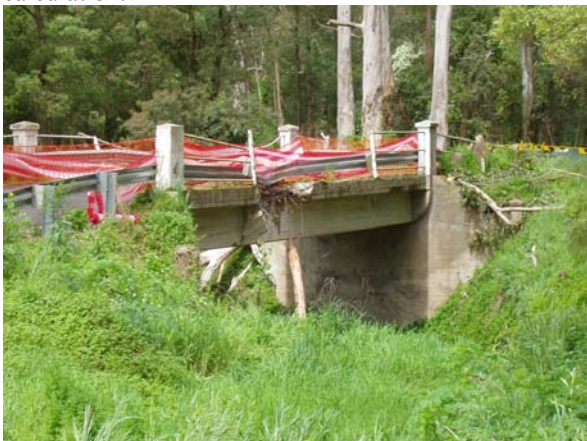
Emergency evaluation of damaged bridge for partial usage
