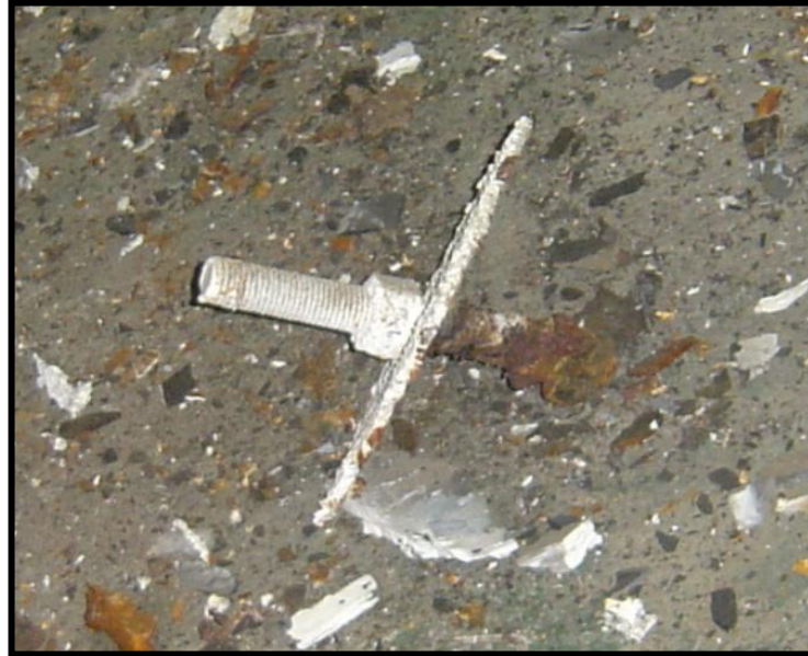
Fig 10 – Corroded bolt, 16 level crib room.
